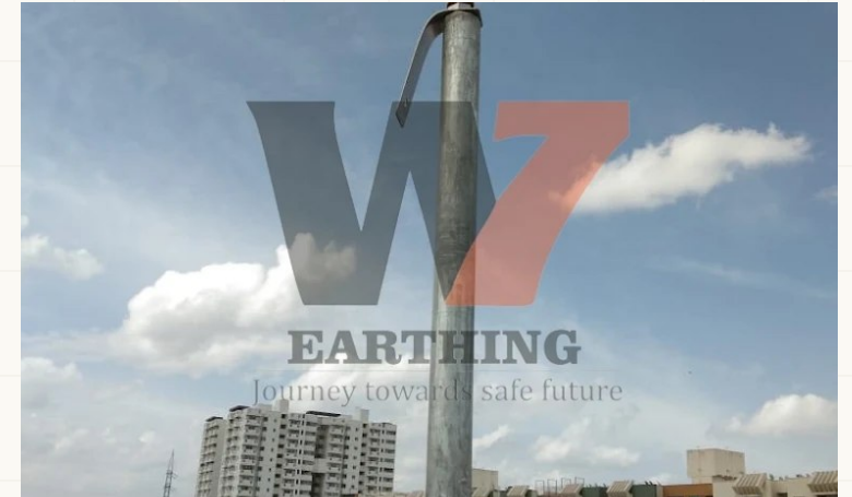
INSTALLED AIR TERMINAL
